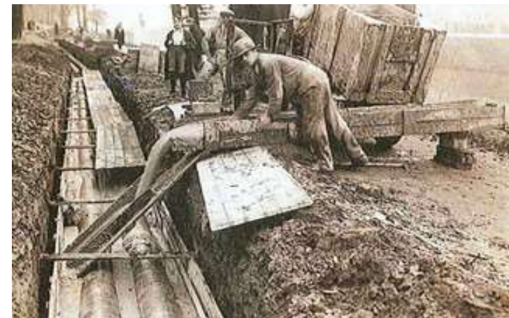
The first network for district heating was constructed in Utrecht to supply heat to the academic hospital at the Catherijnesingel (1923) 10
